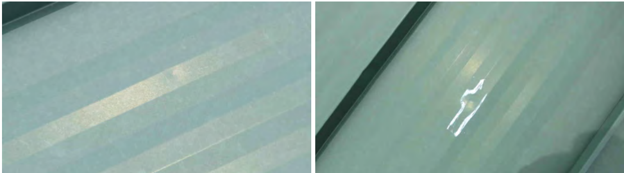
Figure 23. Roofing on the global business development center (5) with hail-related conditions.
