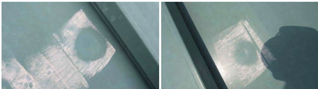
Figure 12. Roofing on the Bob Burns hall (1) with hail-related conditions.
