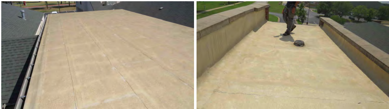
Figure 92. Roofing on the national child protection training center (8) with no wind damage.
