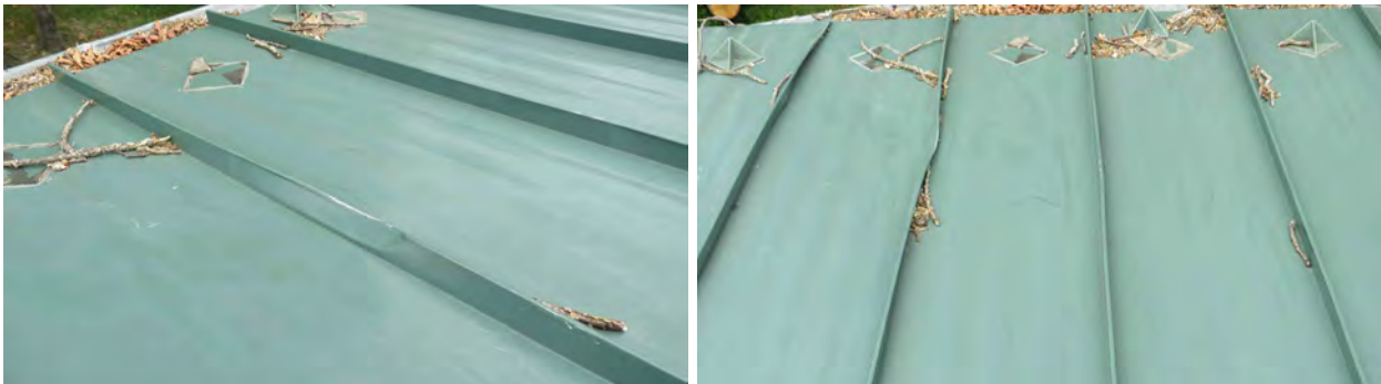
Figure 72. Roofing on the global business development center (5) with wind-related conditions.
