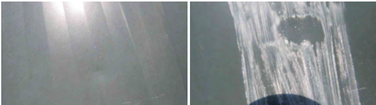
Figure 35. Roofing on the Shrewmaker center for workforce tech (12) with hail-related conditions.
