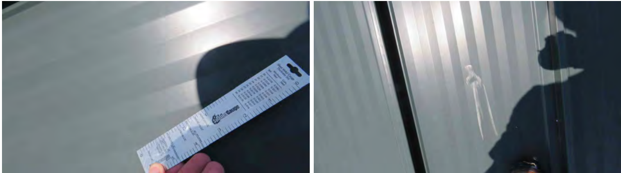
Figure 34. Roofing on the Shrewmaker center for workforce tech (12) with hail-related conditions.
