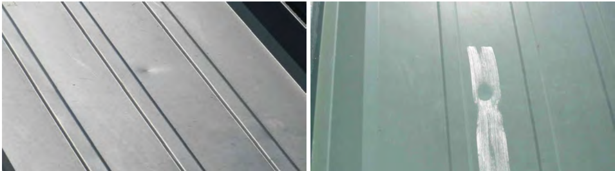
Figure 31. Roofing on the physical plant building (10) with hail-related conditions.
