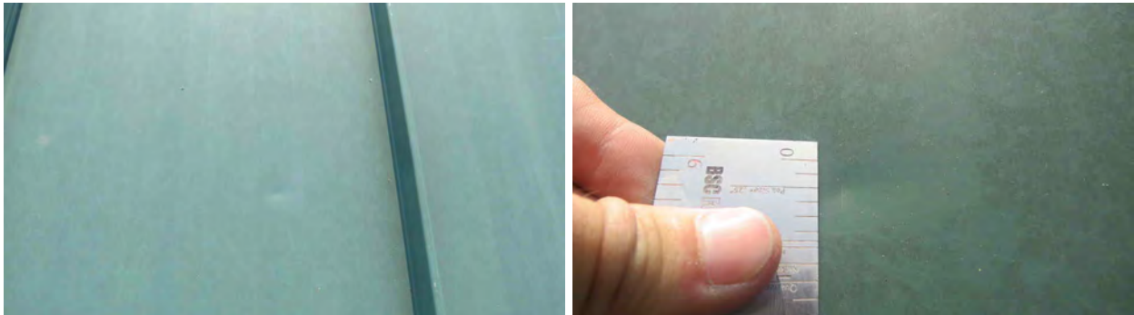
Figure 19. Roofing on the student center (13) with hail-related conditions.
