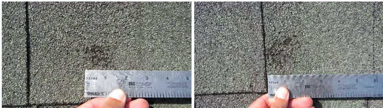
Figure 50. Roofing on the national child protection training center (8) with hail-related conditions.
