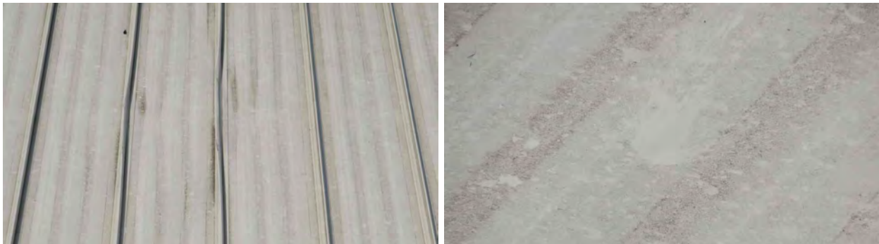
Figure 24. Roofing on the integrated design lab (6) with hail-related conditions.
