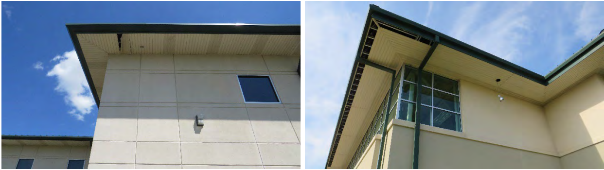
Figure 53. Vulnerable elements at the subject property with wind-related conditions consistent with the reported date of loss.
