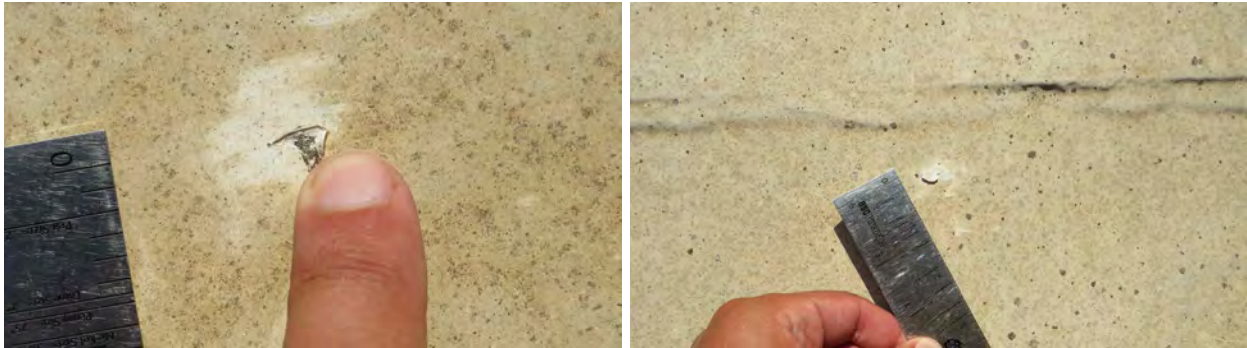
Figure 36. Roofing on the bob burns hall (1) with hail-related conditions.
