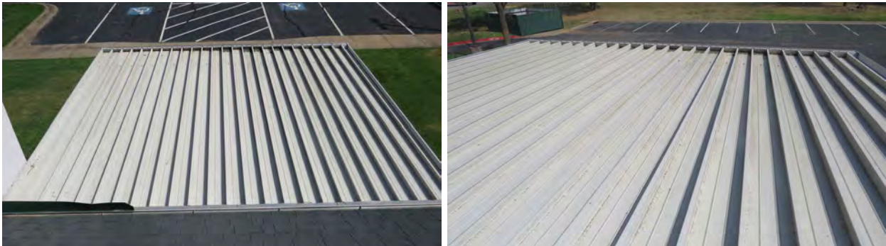
Figure 71. Roofing on the national child protection training center (8) with no wind damage.
