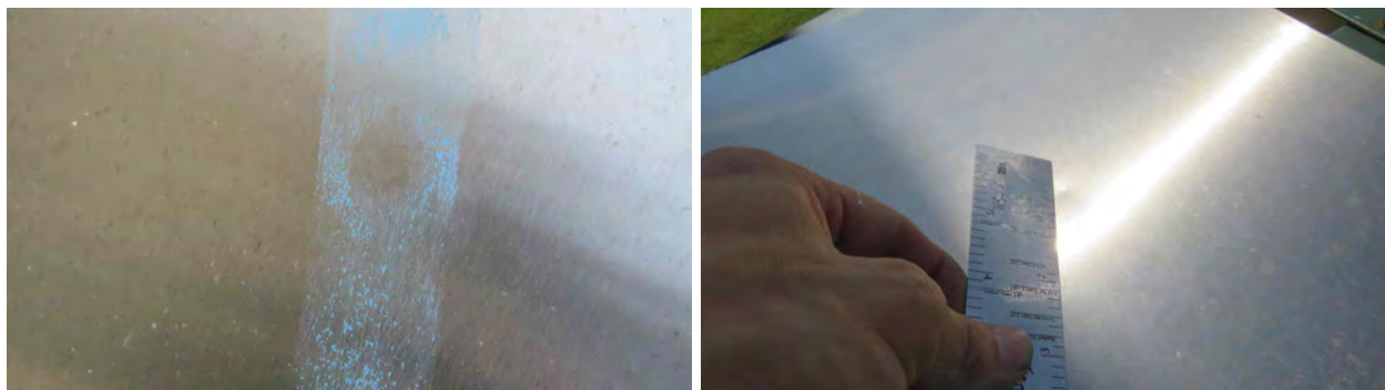
Figure 44. Roofing on the bob burns hall (1) with hail-related conditions.
