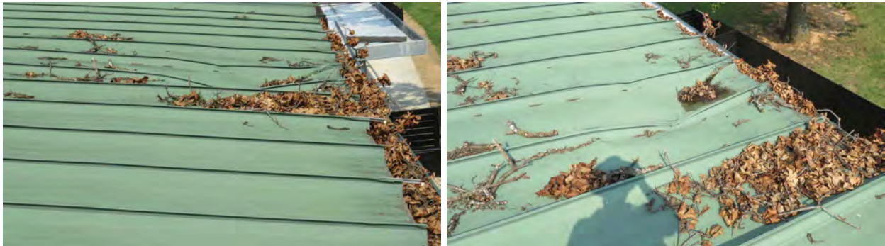
Figure 86. Roofing on the maintenance building (7) with wind-related conditions.
