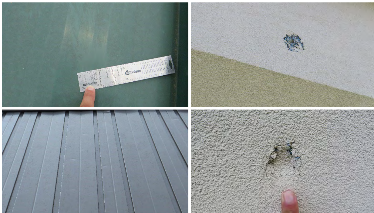
Figure 1. Vulnerable elements with evidence of hailfall consistent with the reported date of loss.
