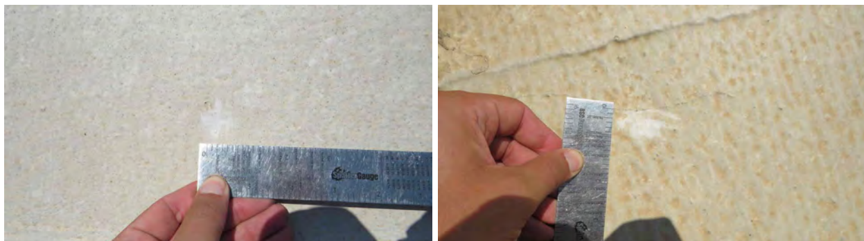
Figure 43. Roofing on the Shrewmaker center for workforce tech (12) with no hail damage.
