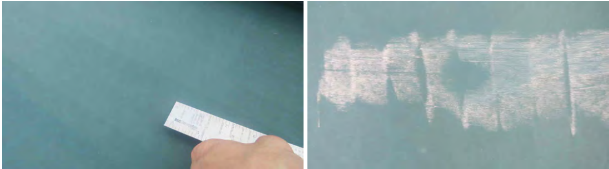
Figure 14. Roofing on the central energy plant (3) with hail-related conditions.
