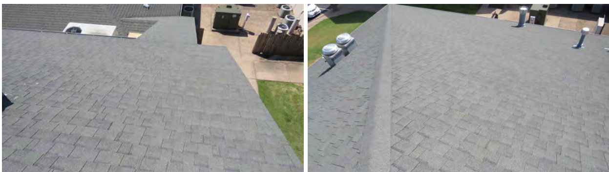
Figure 97. Roofing on the national child protection training center (8) with no wind damage.
