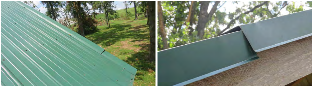
Figure 67. Roofing on the challenge course pavilion (4) with wind-related conditions.
