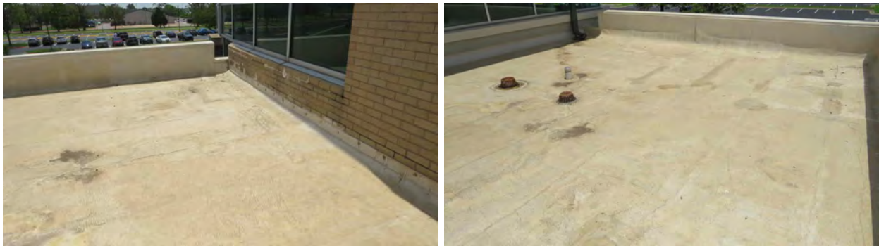
Figure 89. Roofing on the shrewmaker center for workforce tech (12) with no wind damage.
