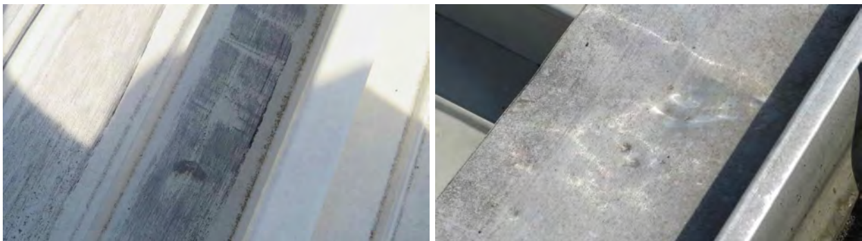
Figure 28. Roofing on the national child protection training center (8) with hail-related conditions.
