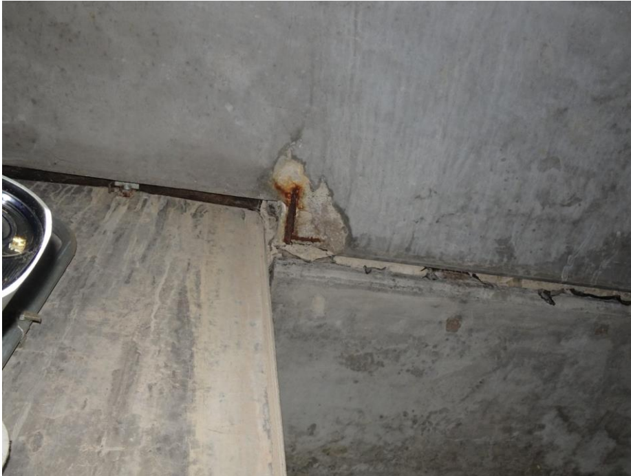
Photo 7. Spalling of double-tee flange with exposed reinforcement.
