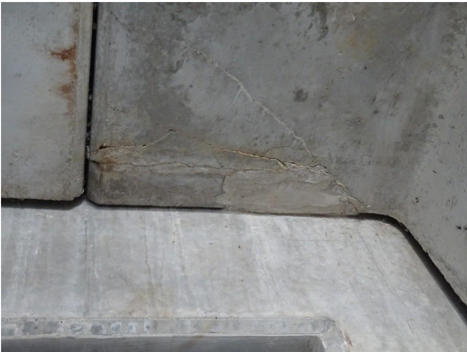
Photo 6. Typical concrete spalling at double-tee flange.
