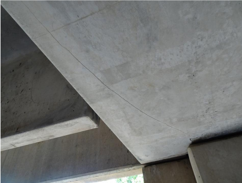
Photo 5. Close-up view of typical cracked inverted-tee girder throughout all levels.
