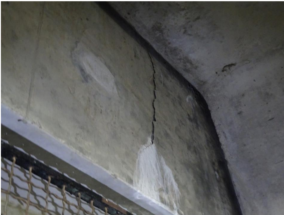
Photo 8. Typical concrete wall spalling.
