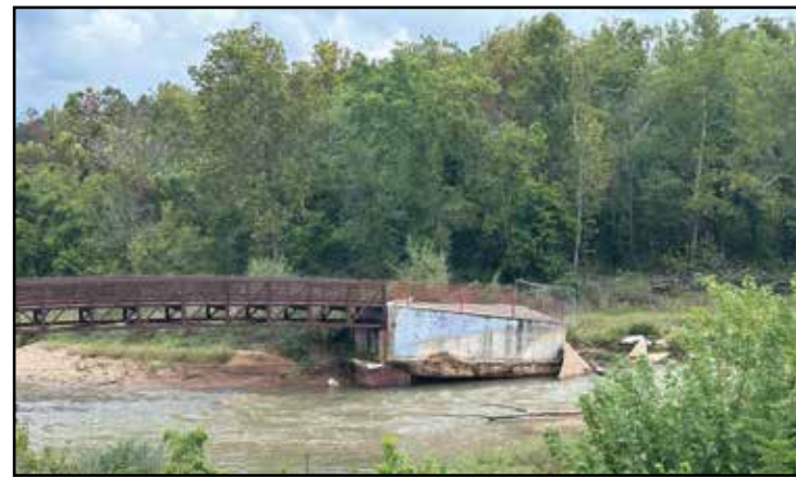
Depicted is the current bridge and erosion that makes the rail unsafe is evident
